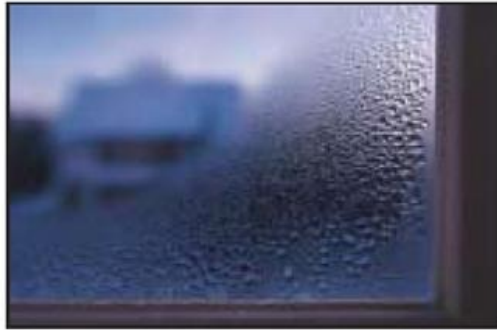
Condensation on the inside of a windowpane.
